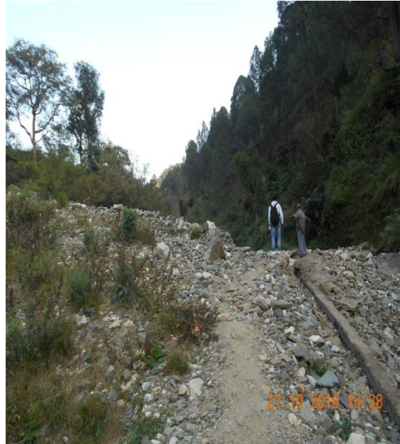
Figure: 1 The road materials moved downward and buried agricultural land in Gir village of Uttarakhand (Photo credit: Author)
